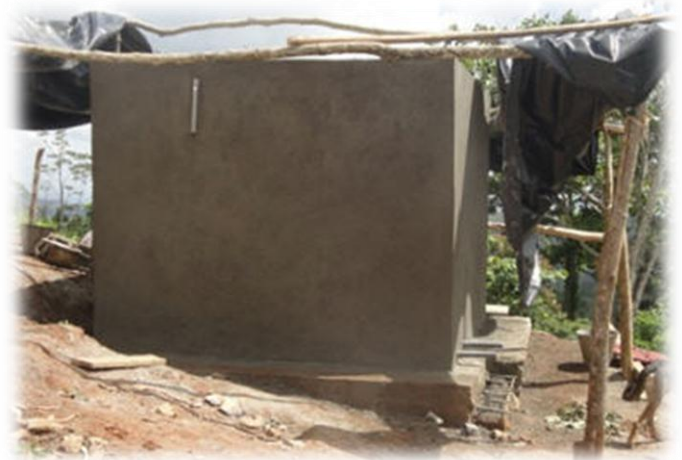
Storage tank at La Esperanza Mar 11, 2011
